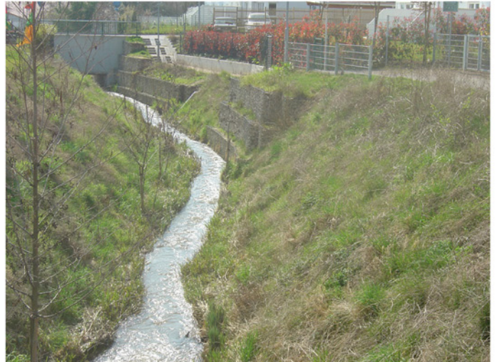
Spring 2007: By the end of the dormant season the whole site is covered with vegetation. The stone revetment underneath is invisible.
