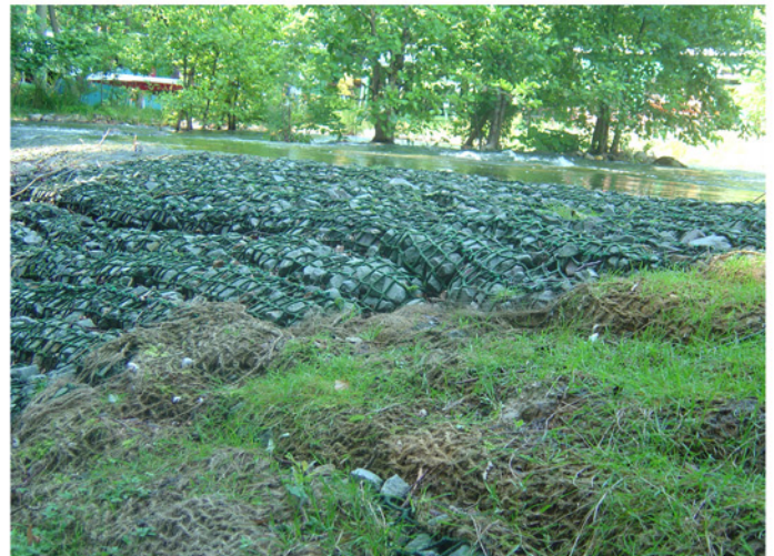
Less frequently overflowed boundaries of the spillway have been covered with coir mesh to improve conditions for sedimentation and to enhance spontaneous cover with greenery.
