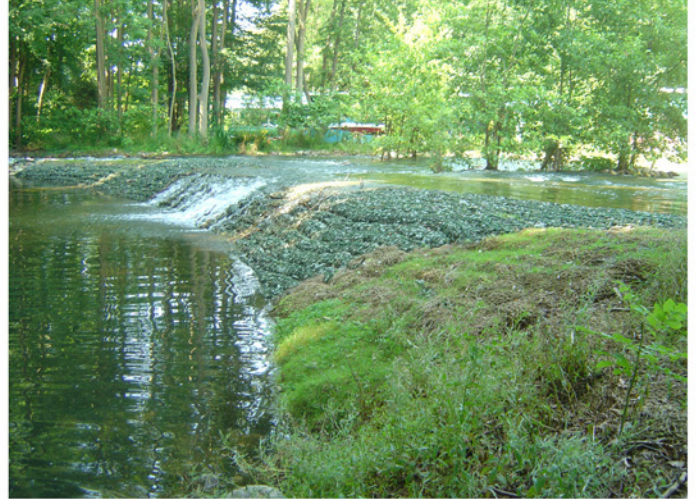
Due to frequent floodwater discharges the spillway has been exposed to permanent overflow in summer 2007.
