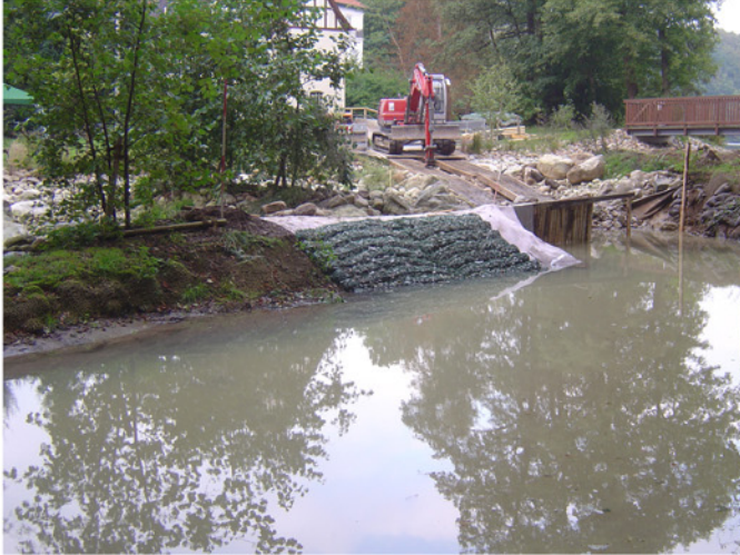
The rock mattresses have been installed on a filter cloth in summer 2006.
